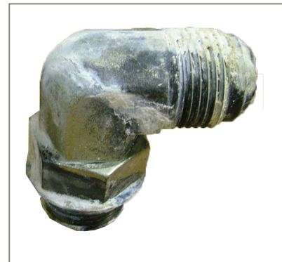
Figure 5: Zinc Oxidation on a Steel Tube Fitting
