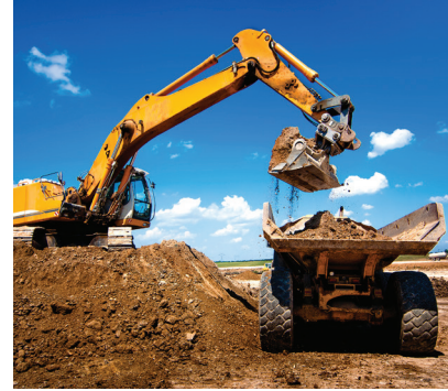
Figure 2: Corrosion can quickly develop on off-road equipment even in normal environmental conditions
